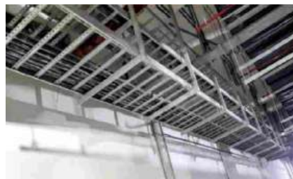
Cable Trays & Raceways
