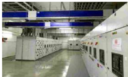
Sandwich Bus Ducts & LT Panels
