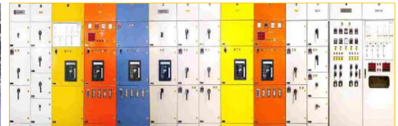
EPC Contracts : Substations, DG Sets, Lighting, Wirings, Cables, Cable Trays.
